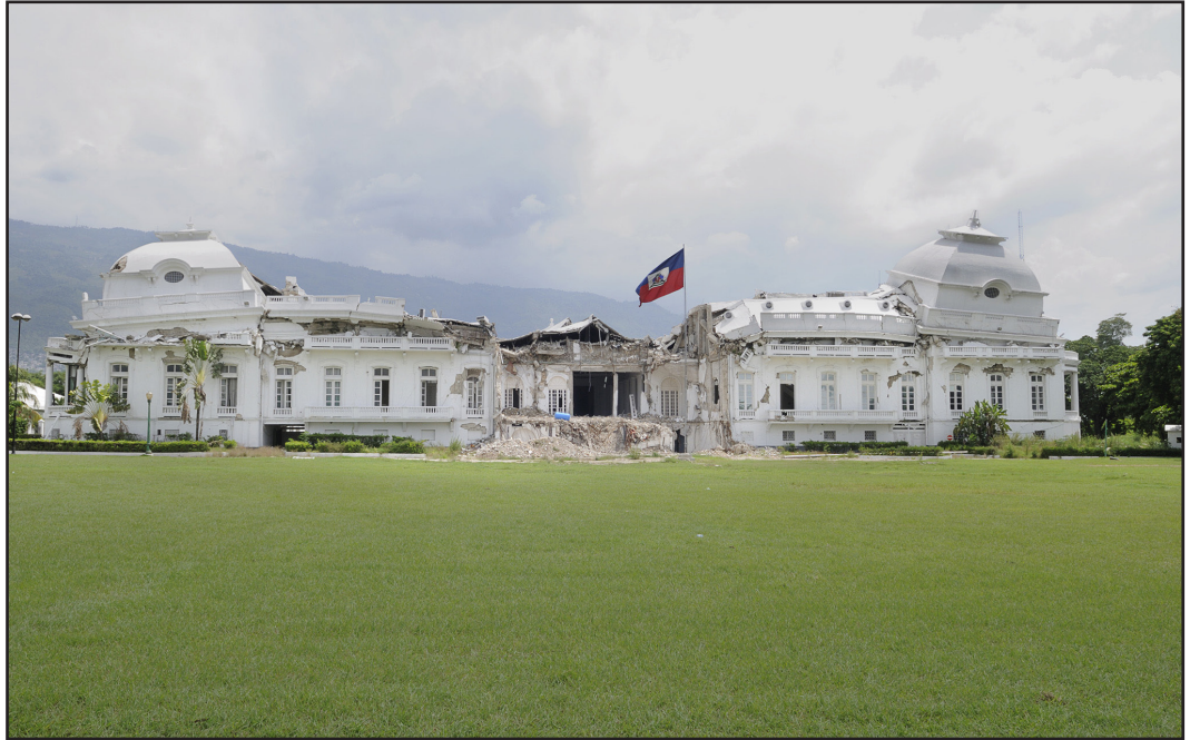
The Haitian National Palace (Presidential Palace), located in Port-au-Prince, Haiti, heavily damaged after the earthquake of 12 January 2010.
